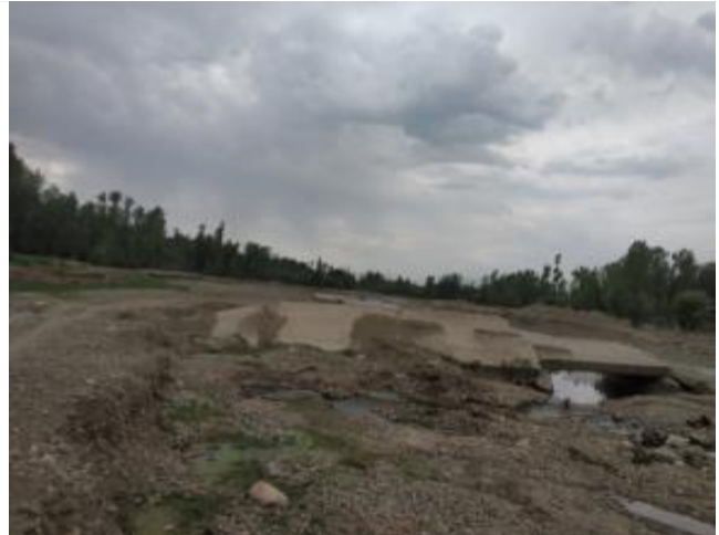
Odds and ends of the damaged bridge (which was washed away during 2014 floods) near proposed bridge site downstream.
