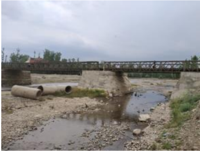
Existing temporary bailey bridge on RHS of the proposed bridge. This temporary was constructed after 2014 floods and was damaged number of times.
